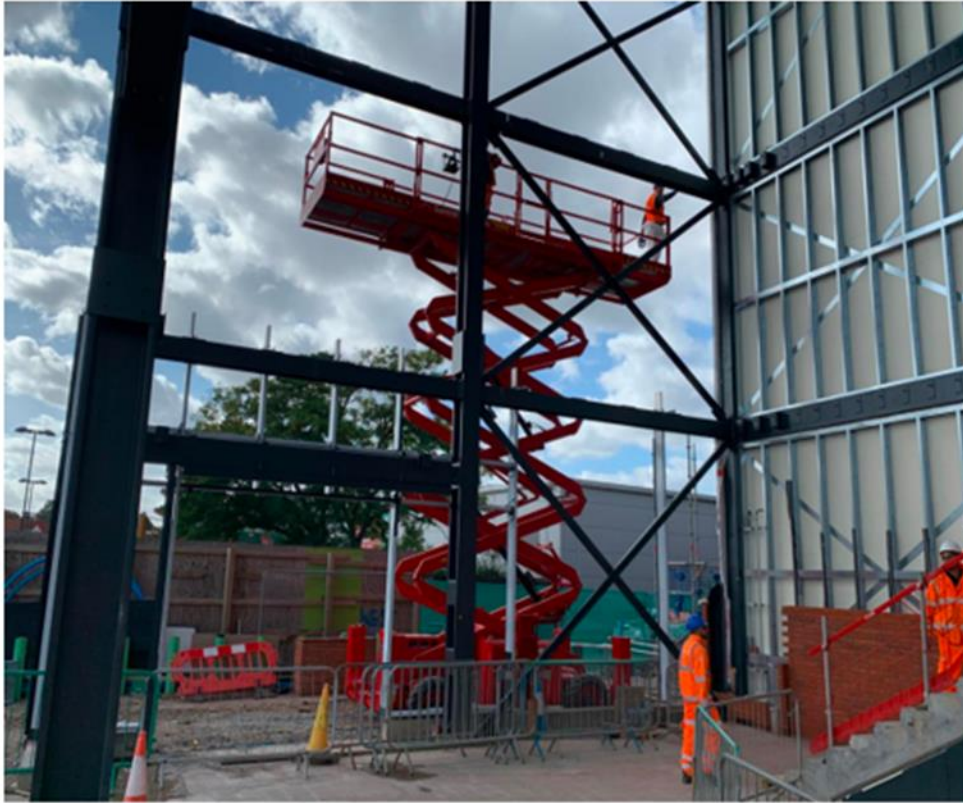
WEB curtain wall mullions and paint touch ups in progress Internal brickwork first lift installed to the north elevation
