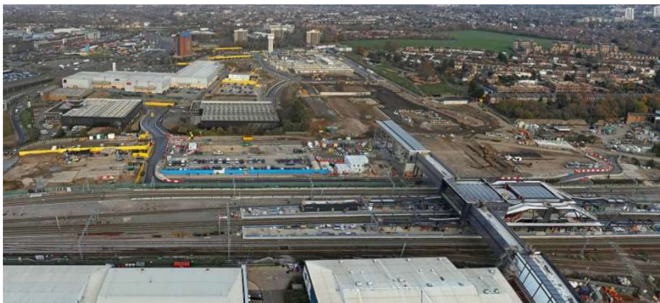
Brent Cross West Station in the foreground. Brent Cross Town in the background (December 22)
