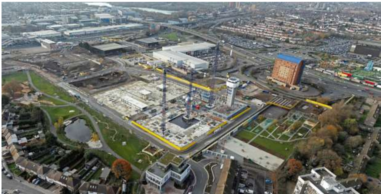
First tower cranes constructed and core of plot 12 now visible above ground (December 22)
